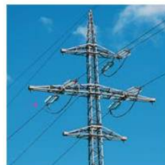
Fig. 13 Pylon for electric power lines.
